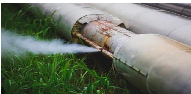
Plate 1: pipeline gas leakage scenario ( http://www.shutterstock.com )
